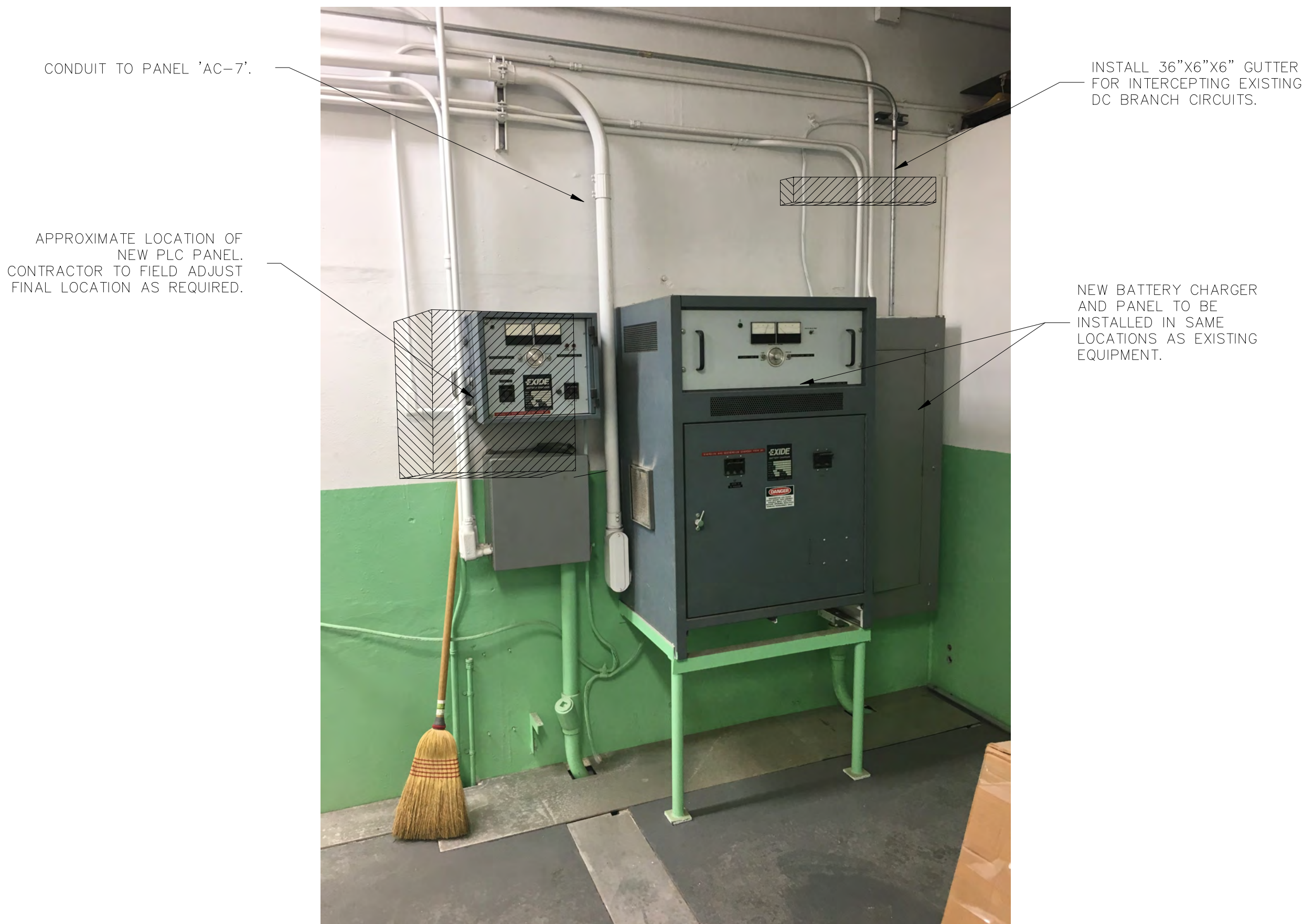
PICTURE 4: OLD POWERHOUSE DC EQUIPMENT
