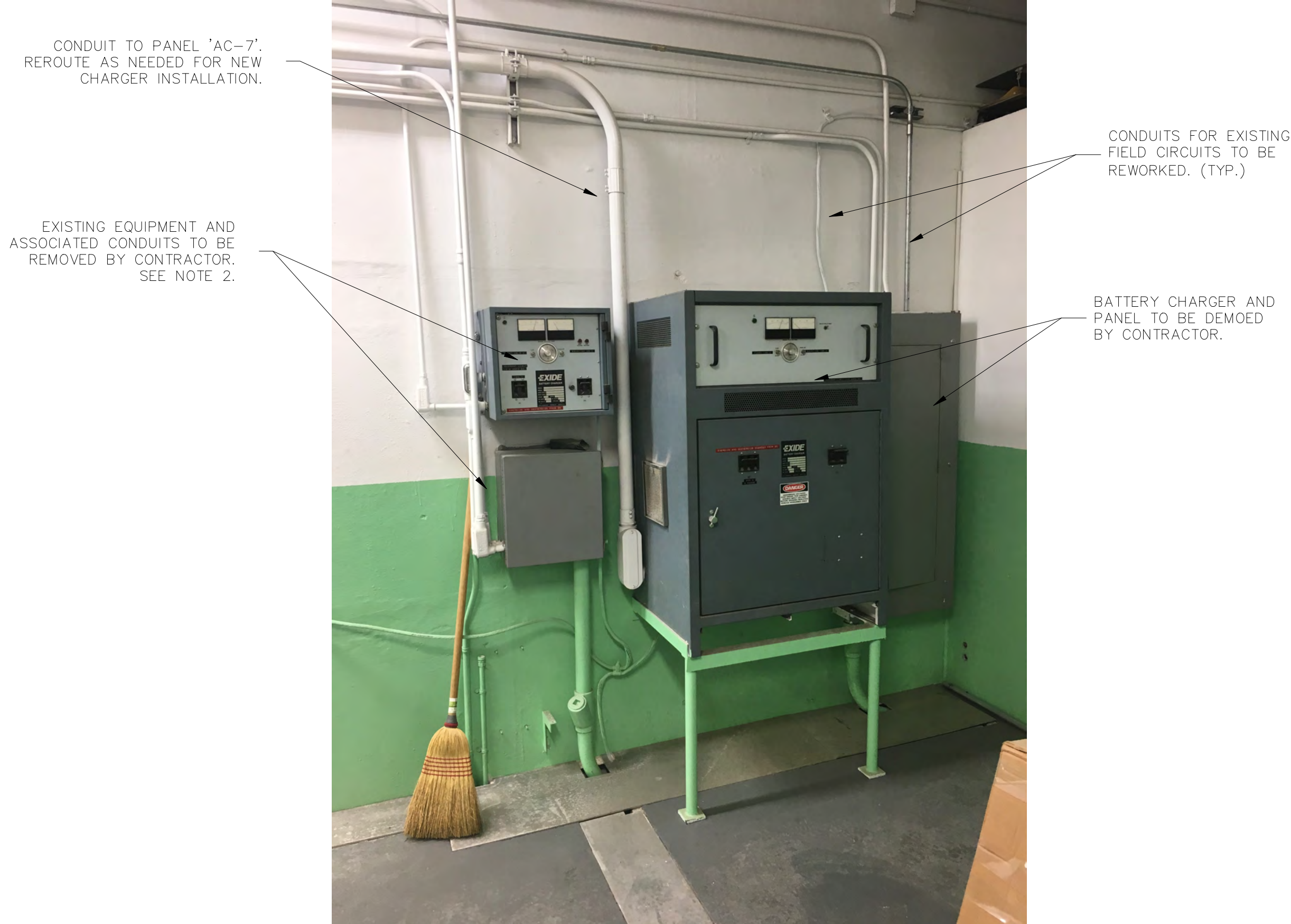
PICTURE 4: OLD POWERHOUSE DC EQUIPMENT – DEMO
