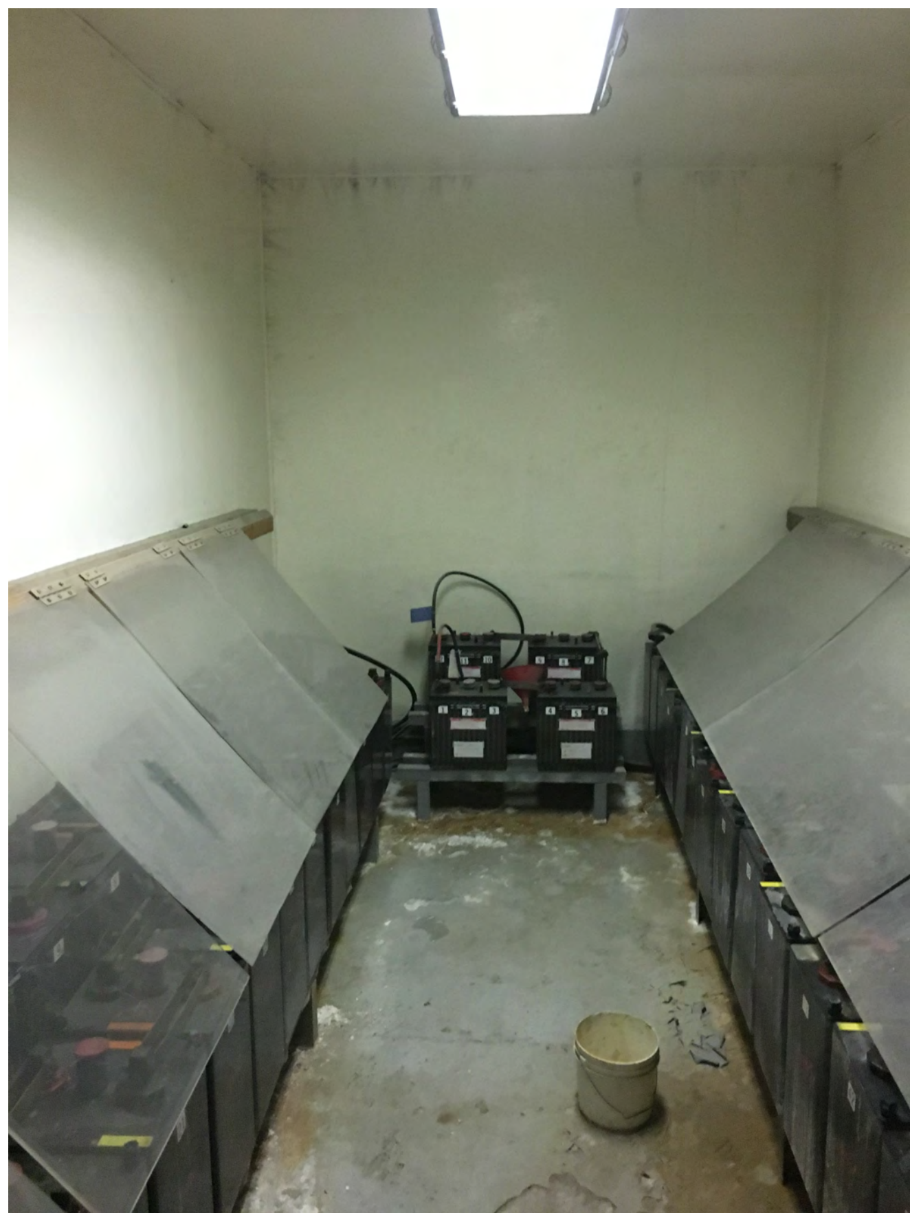
PICTURE 1: BATTERY ROOM
