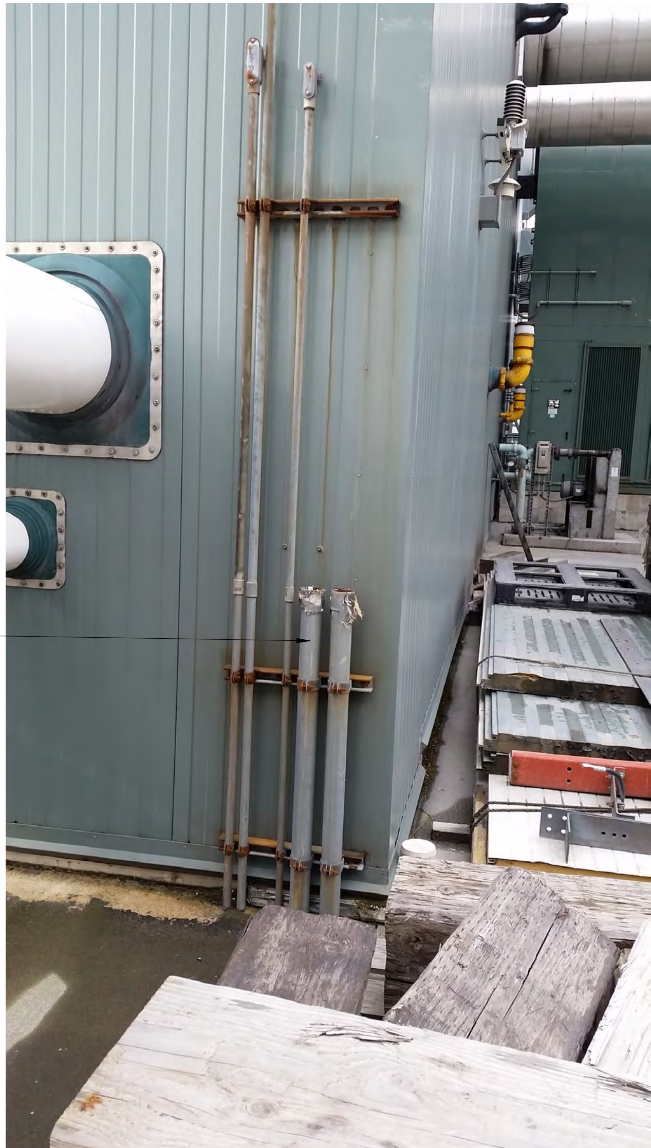
PICTURE 1: NEW POWERHOUSE SPARE CONDUITS
