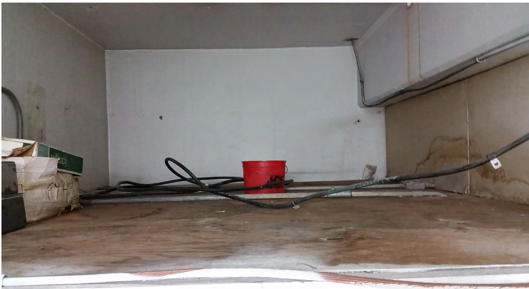
PICTURE 2: BATTERY ROOM CEILING
