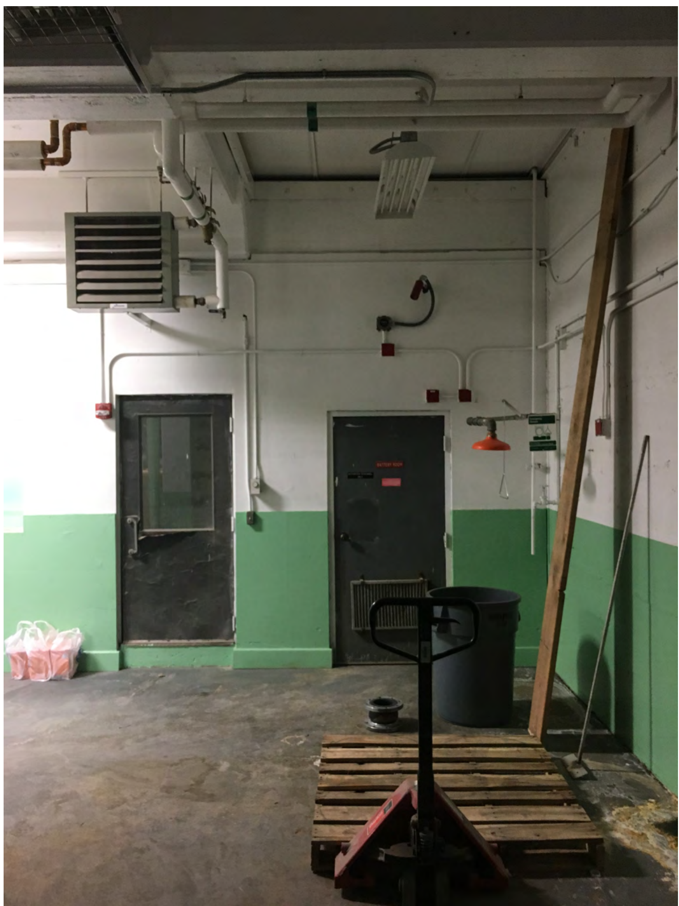
PICTURE 3: OLD POWERHOUSE BATTERY ROOM ENTRANCE
