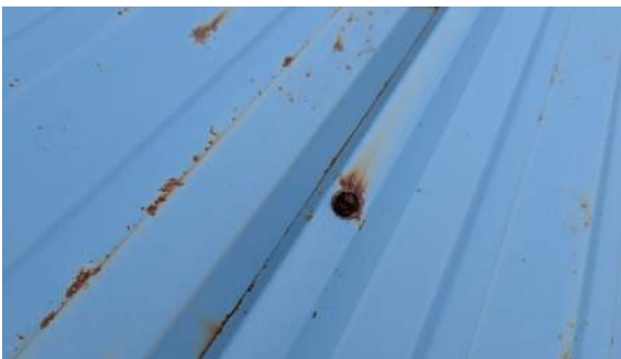
Photo #5: Hex head fasteners in the standing seams are rusted. Gaskets are either missing or cracked.
