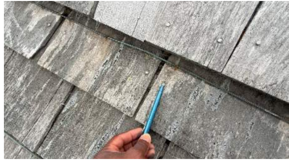
Photo #10: Exposed fasteners
