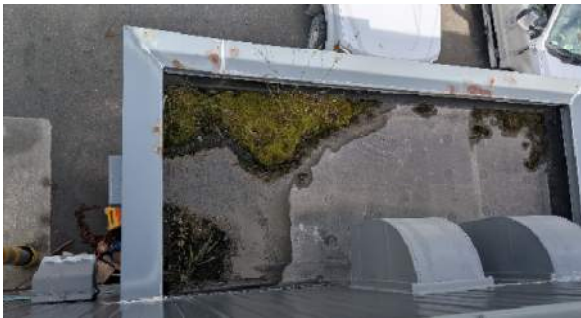
Photo #5: Moss and grass growing on lower roofs causing ponding
