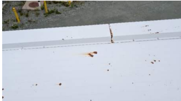
Photo #2: Eave of roof panels are rusting.
