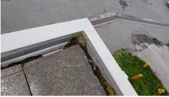
Photo #1: Moss and grasses growing between coping and pavers along entire roof.
