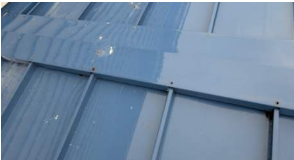
Photo #45: Missing fasteners on ridge flashing
