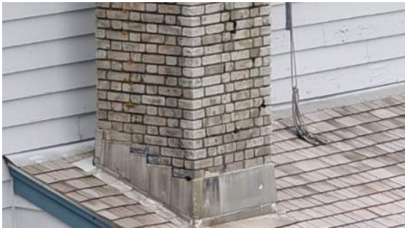
Photo #5: Roof to wall flashing at entrance is missing.
