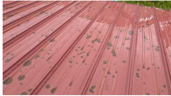
Photo #2: Large rust spots covering entire corrugated metal roof, continued
