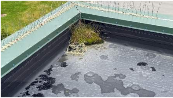
Photo #1: Grass and vegetation growing on cedar and membrane roofing
