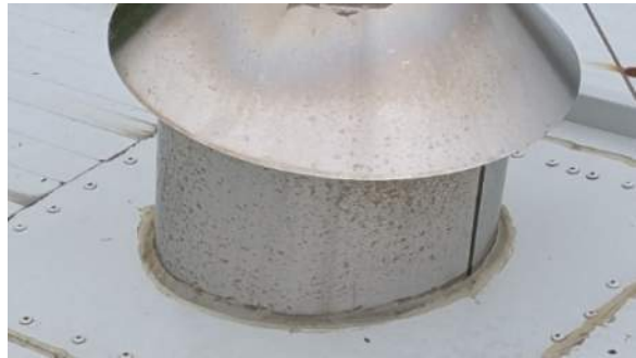
Photo #4: Sealant pulling away from chimney flashing.
