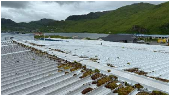
Photo #41: Moss at roof ridge
