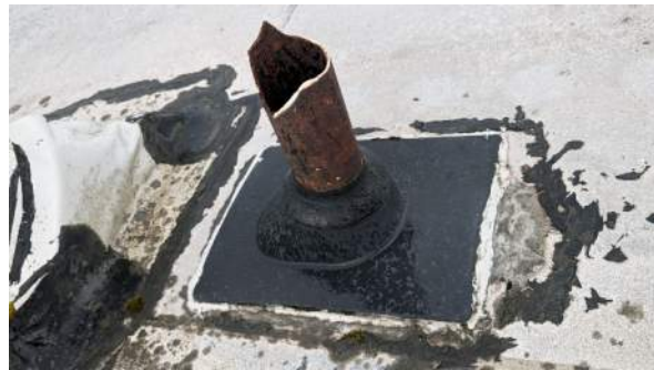
Photo #29: Boot at vent through roof sealant has failed and is pulling away. Steel pipe is also broken
