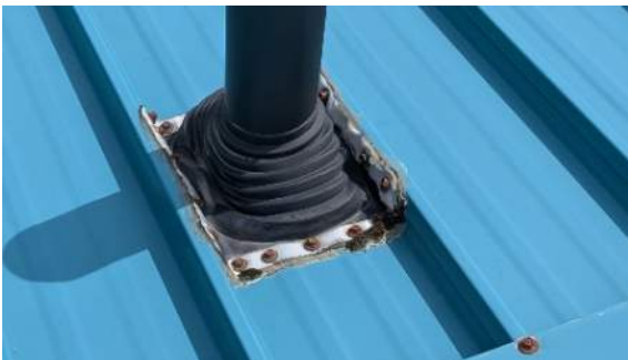
Photo #7: Moss growing on sealant.
