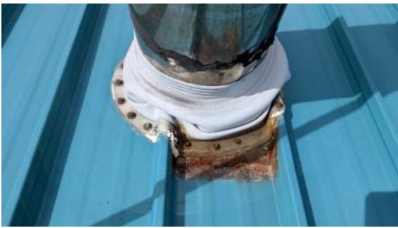
Photo #3: Heavy rust. Sealant is no longer providing any protection.
