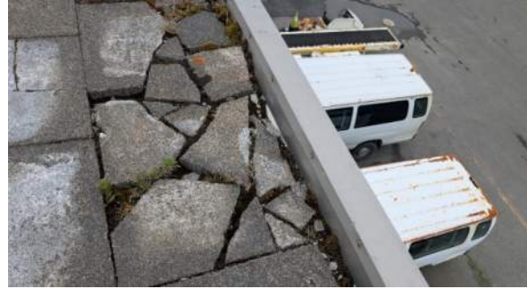
Photo #2: Broken pavers in multiple locations across entire roof.
