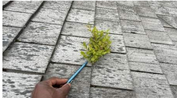
Photo #2: Grass and vegetation growing on cedar and membrane roofing, continued
