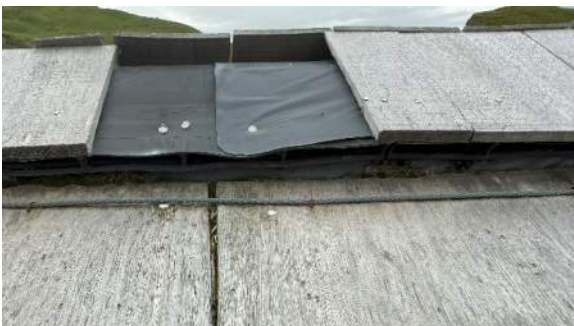
Photo #5: Cedar shakes on roof missing
