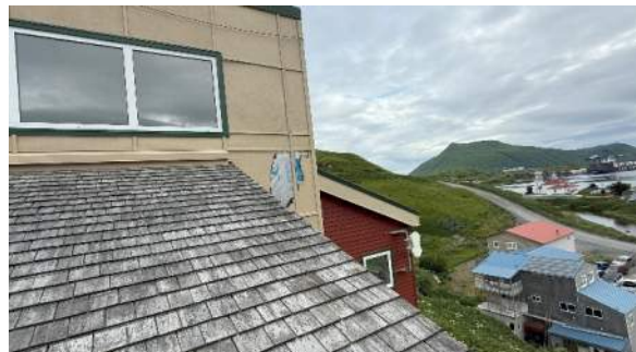
Photo #8: Section of exterior wall torn off
