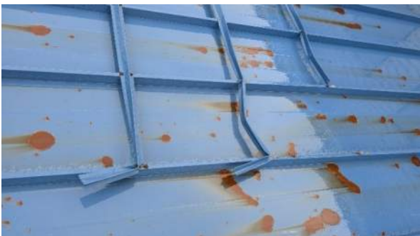
Photo #49: Snow guard bent or broken
