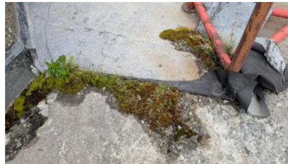
Photo #3: Moss and lichen growing on roof in spots.
