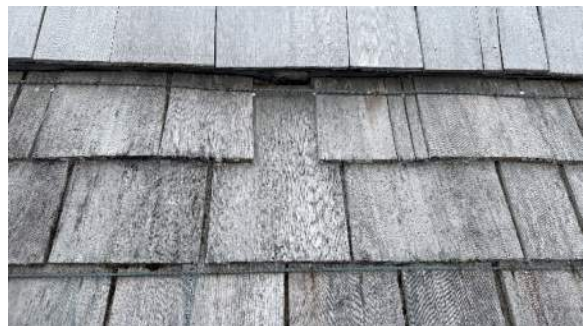
Photo #6: Cedar shakes on roof missing, continued
