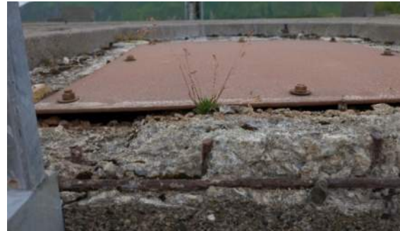
Photo #1: Edge of concrete roof crumbling with exposed rebar.
