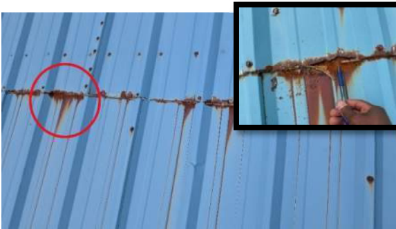
Photo #3: Edges where corrugated sheets overlap have rusted away. Sealant at these locations is attached to nothing at this point.
