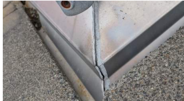
Photo #6: Broken sealant.
