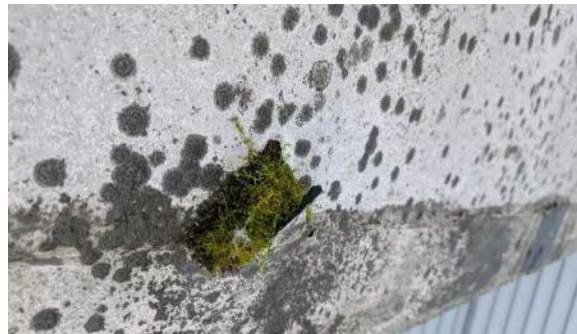
Photo #30: Moss and grass grow in the holes in the roof membrane
