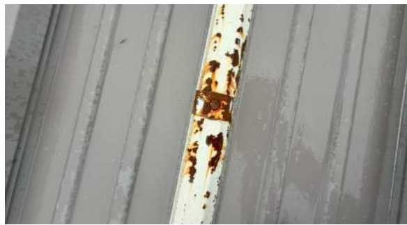
Photo #12: At missing rib cover, the rib and fastener are heavily rusted.
