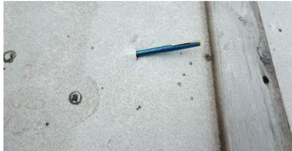
Photo #32: Holes in membrane
