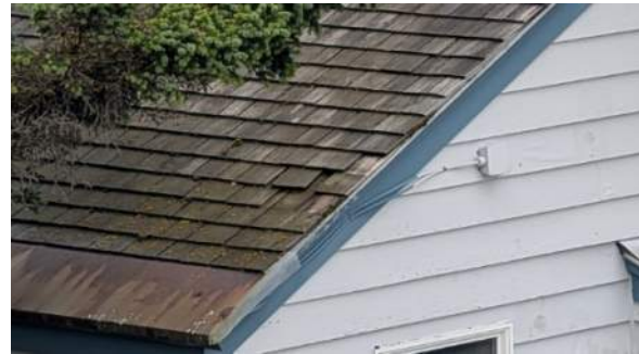
Photo #2: Missing Cedar shakes.
