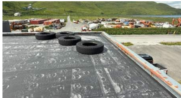
Photo #6: Perimeter membrane failure at roof corner. Weighted down with tires.
