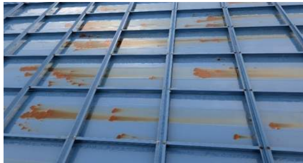
Photo #46: Rust spots all over metal roofing
