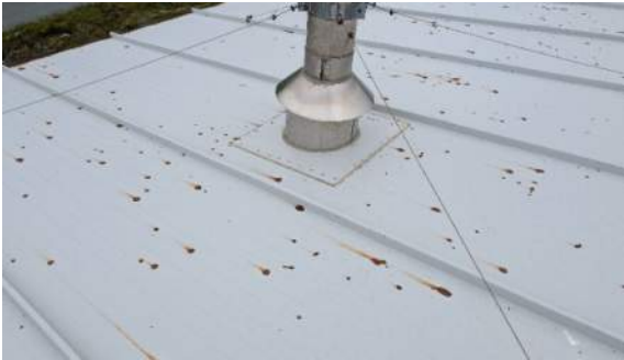
Photo #1: Rust spots across the entire roof.
