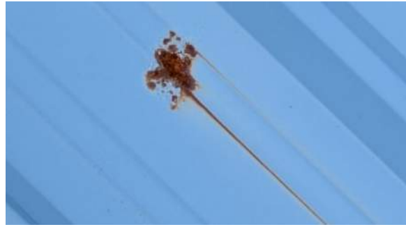
Photo #2: Portions of the metal roofing have severe rust spots causing holes.
