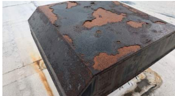
Photo #27: Exhaust hood is rusted
