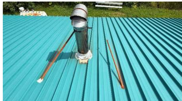
Photo #8: Broken and rusted chimney stay rods.
