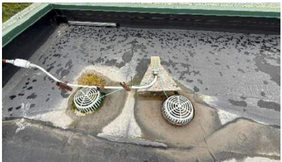
Photo #13: Hazardous conduit location
