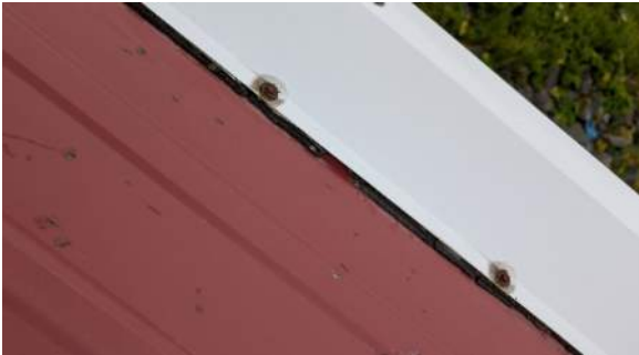
Photo #3: Exposed fasteners at panel laps
