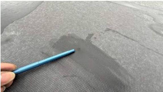
Photo #3: Protruding object under the membrane roof. High wear point, potential puncture hazard
