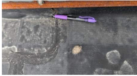
Photo #2: Roof membrane patched in multiple spots. Some have started to peel away.
