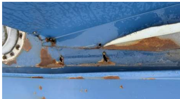
Photo #50: Fasteners torn out of metal roofing
