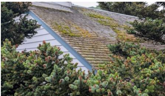
Photo #3: Roof is growing moss, grass and lichen.
