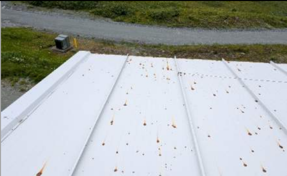
Photo #6: Rust spots across the entire roof, continued
