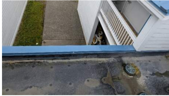
Photo #38: Moss and grass growing in roof gutter. Ponding between roof and overflow and roof drain, continued
