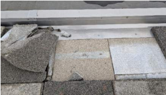
Photo #5: Exposed flashing.
