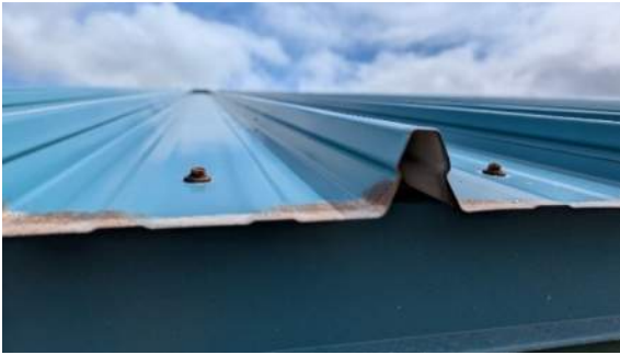
Photo #1: Roof eave is rusting. Fasteners are rusting.
