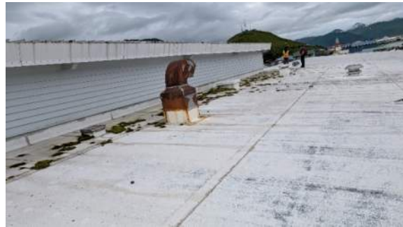
Photo #28: Exhaust hood is rusted, continued
