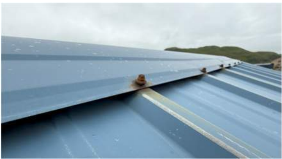
Photo #3: Ridge closer is missing. Fasteners are heavily rusted. Flashing rusting beneath. Gaskets are missing or deteriorating.
