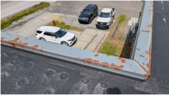
Photo #1: Coping rusting. Largely at connections and lapping.
