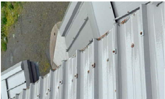
Photo #5: Roof eave paint is peeling away and starting to rust.
