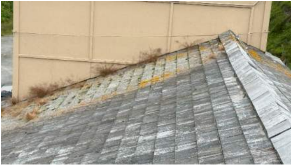
Photo #11: Lichen stains at shingle field
