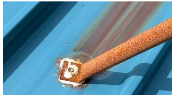
Photo #4: Rusty support has leached onto roof. Rust has formed beneath.
