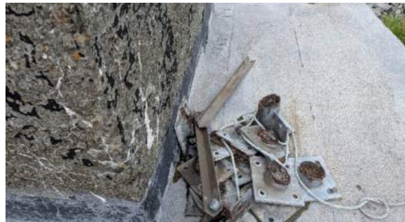
Photo #4: Areas of roof have roofing material covering concrete roof. You can feel crumbling roof underneath.
