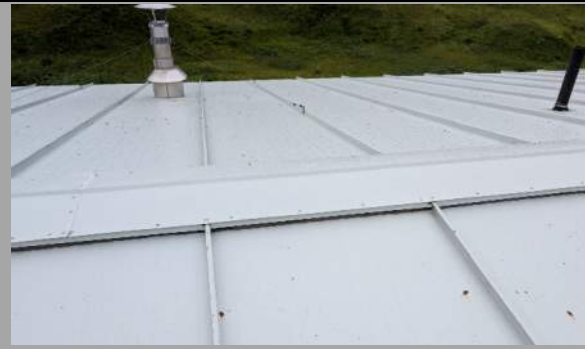
Photo #7: Fastener backing out.
