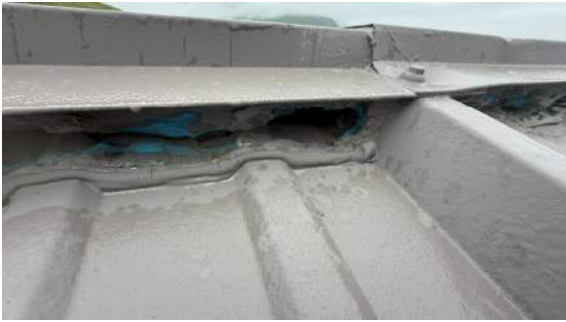
Photo #7: Foam closer in multiple locations has been picked out by birds leaving holes that provide no protection
