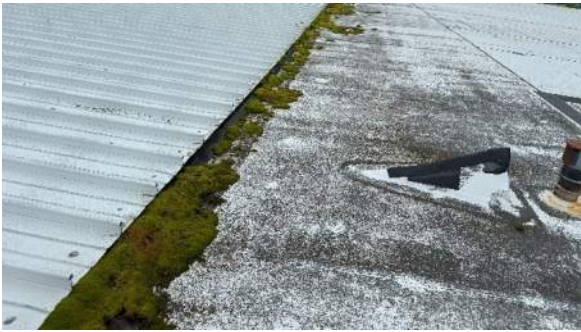
Photo #39: Moss and lichen at roof
