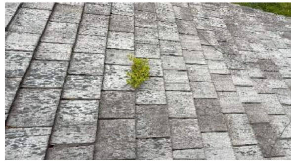
Photo #14: Grass and vegetation growing on cedar and membrane roofing, continued
