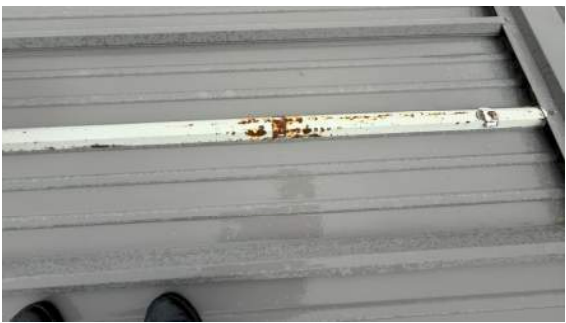
Photo #11: Multiple roofing rib covers missing, shifting or coming off.
