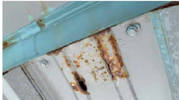
Photo #10: Roof panel at eave has hole rusted into it.
