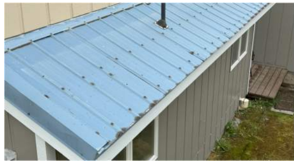
Photo #4: Ridge closer is missing. Fasteners are heavily rusted. Flashing rusting beneath. Gaskets are missing or deteriorating. Spots on the eave are starting to form rust.
