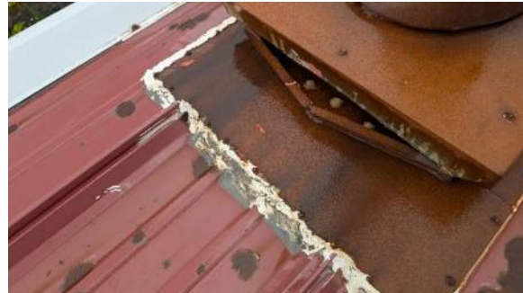
Photo #6: Rusted chimney hood and base, sealant starting to pull away, continued
