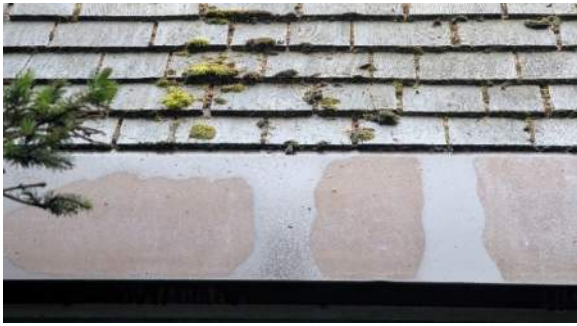
Photo #1: Galvanized metal eave flashing is rusting.
