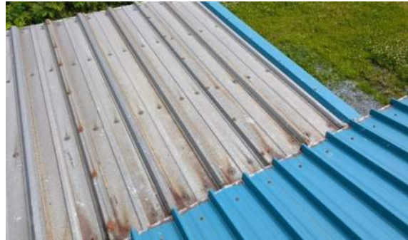
Photo #8: Roof and fasteners are rusting. Rust along main roof edge, continued.
