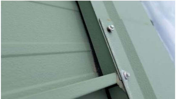
Photo #10: Non NRCA flashing lap
