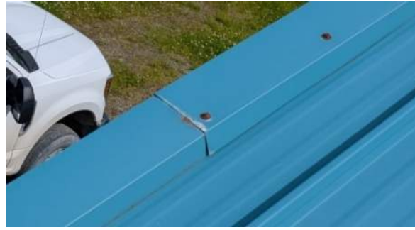
Photo #2: Rust forming where edge flashing overlaps.
