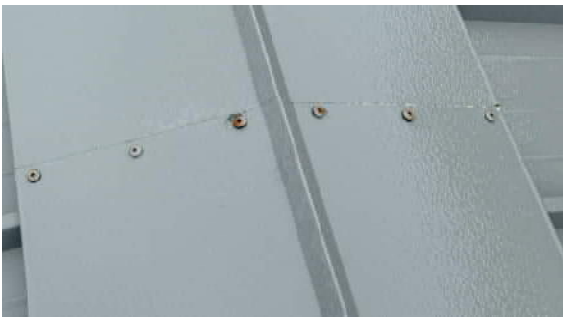
Photo #3: Rib fasteners and clamps are starting to rust. Ridge cap paint is starting to chip at fasteners.
