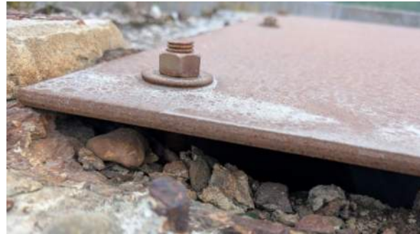
Photo #2: Rusted steel plates over openings. Edges of openings underneath are crumbling in.
