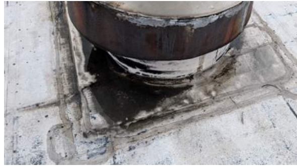
Photo #25: Sealant is failing and has failed around roof penetrations, vents, and snow triangles, continued
