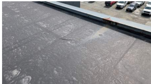
Photo #4: Wrinkles in membrane roofing.
