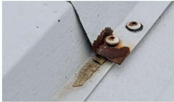
Photo #5: Fastener backing out.
