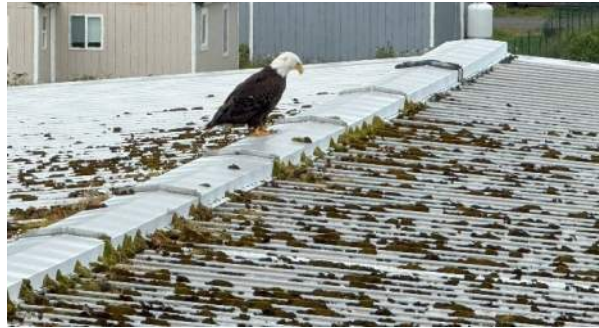
Photo #44: Moss growing on metal roof
