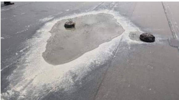
Photo #3: Water ponding around roof drains & grass growing
