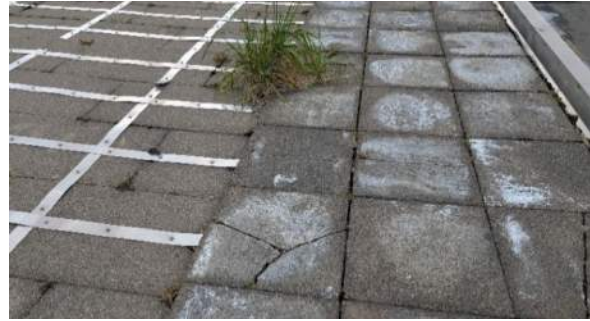
Photo #4: Moss and grass growing between pavers, continued.
