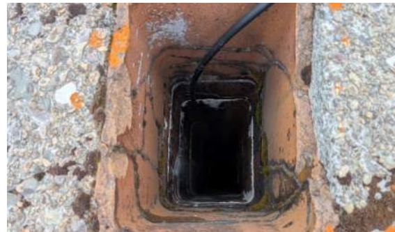
Photo #5: Damaged chimney lining.
