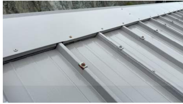
Photo #2: Rib fasteners and clamps are starting to rust.
