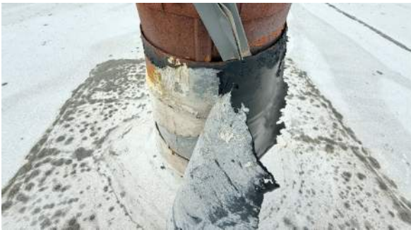
Photo #35: Sealant peeling away at exhaust vents
