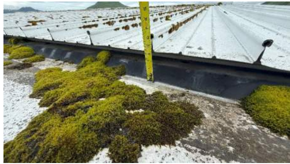
Photo #40: Degraded gasket
