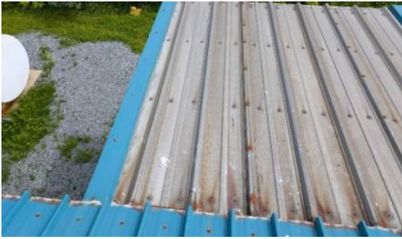
Photo #7: Roof and fasteners are rusting. Rust along main roof edge.
