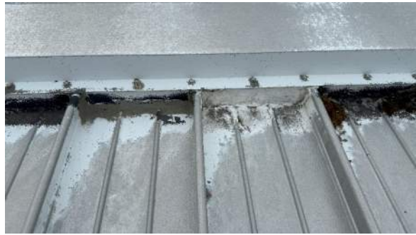
Photo #42: Previous repairs at roof closures
