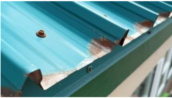
Photo #5: Rusty support has leached onto roof. Rust has formed beneath.
