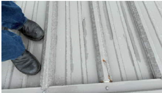
Photo #9: Rib cover is rusting and causing paint to peel.
