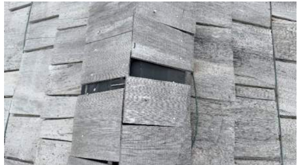
Photo #4: Cedar shakes at ridge broken or missing
