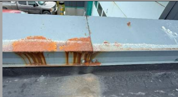
Photo #6: Corrosion at coping
