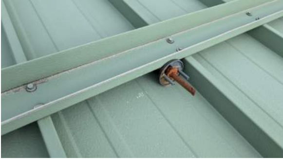
Photo #7: Rusty doorknob on roof. Removed.
