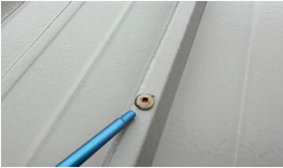
Photo #1: Some square head fasteners gasketed are starting to root.
