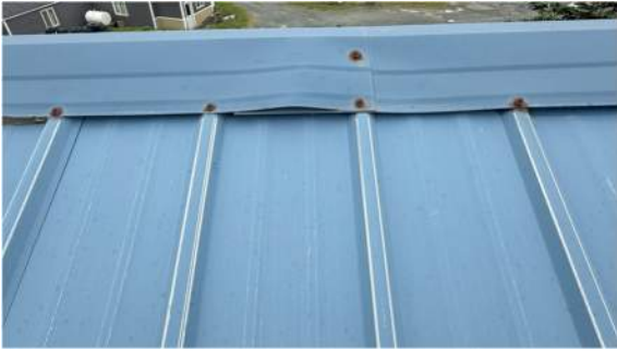
Photo #1: Warped ridge flashing.
