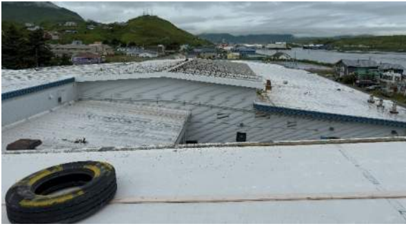
Photo #43: Moss growing on metal roof
