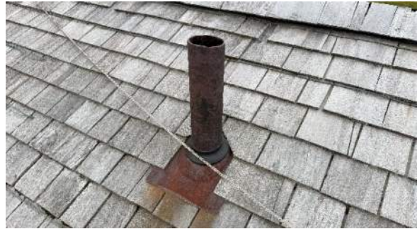
Photo #12: Deteriorated pipe flashing
