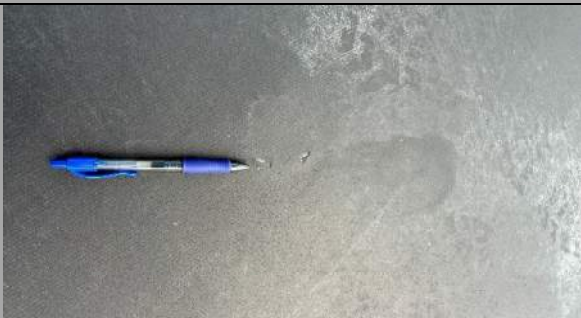
Photo #5: Hole in membrane
