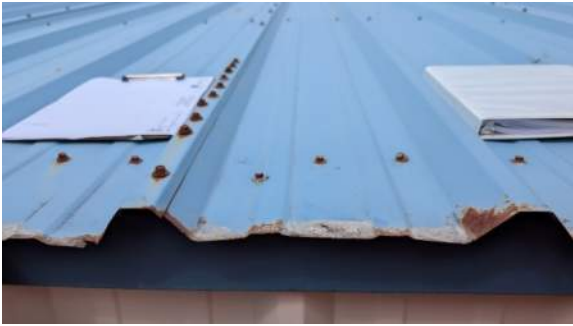
Photo #1: Metal roof edge is rusting and weakening.
