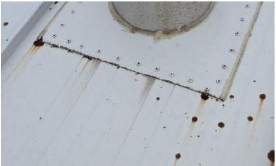
Photo #5: Pitted rust spots at chimney flashing to roof.
