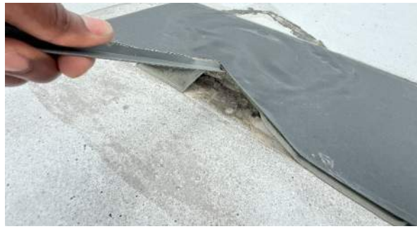
Photo #36: Roof patch has failed
