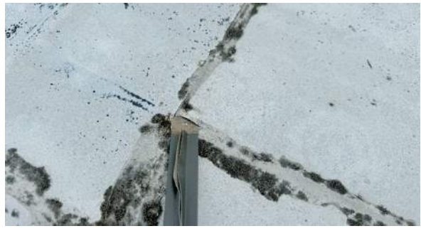
Photo #34: Open Seam at Membrane Lap
