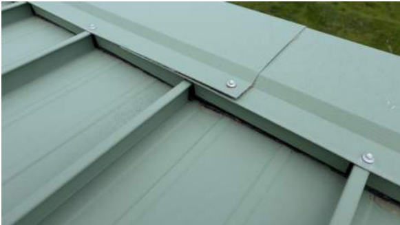
Photo #9: Hex head fasteners have backed out or are not installed properly. Locations include: valleys, ridges, and edge flashings, continued
