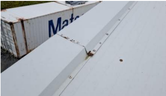
Photo #3: Gaps between edge flashings.
