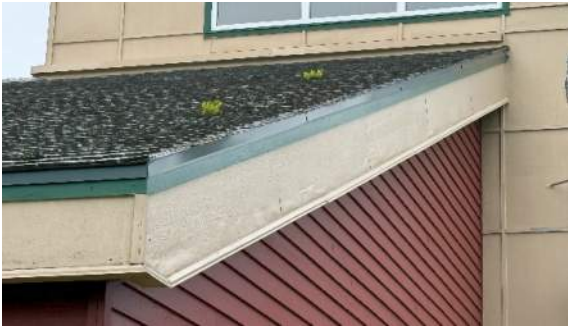
Photo #9: Grass and vegetation growing on cedar and membrane roofing
