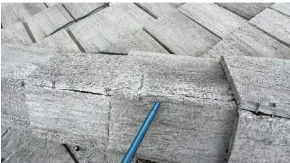
Photo #7: Cedar shakes on roof damaged
