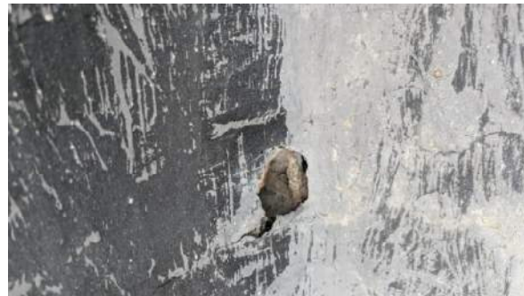
Photo #6: Roofing material damaged, holes, pulled away and destroyed.
