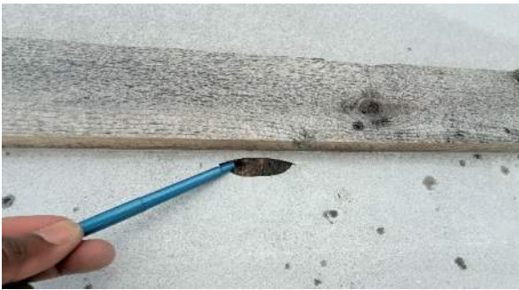
Photo #33: Hole in Membrane
