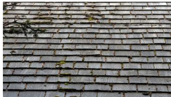
Photo #4: Roof is growing moss, grass and lichen.
