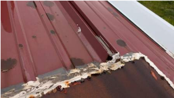
Photo #5: Rusted chimney hood and base, sealant starting to pull away
